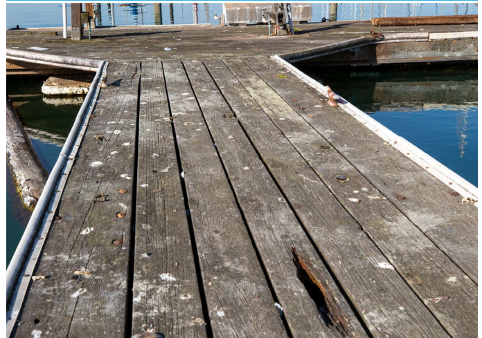
Deteriorated Marina Dock
