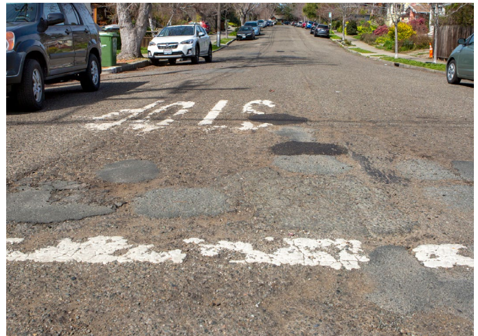
Street Pavement Damage
